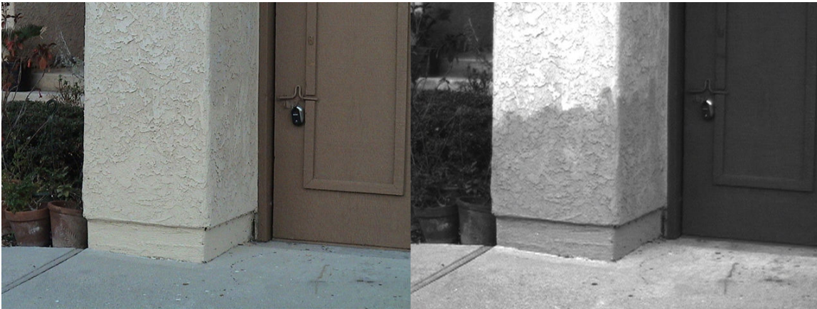
Figure 9. Freshly repainted stucco exterior wall. The fresh paint is dark in appearance. Left – color, right – near-UV
