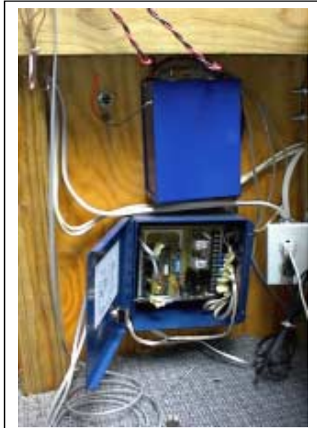
DDW Observatory Control System (12V dome power supply above)
